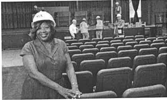
Lorna Lewis, superintendent of the Plainview-Old Bethpage school district, in the auditorium of Stratford Road Elementary School in Plainview on Aug. 10, with construction underway on the air-conditioning and sound systems. New seating also was installed. Photo Credit: Corey Sipkin
